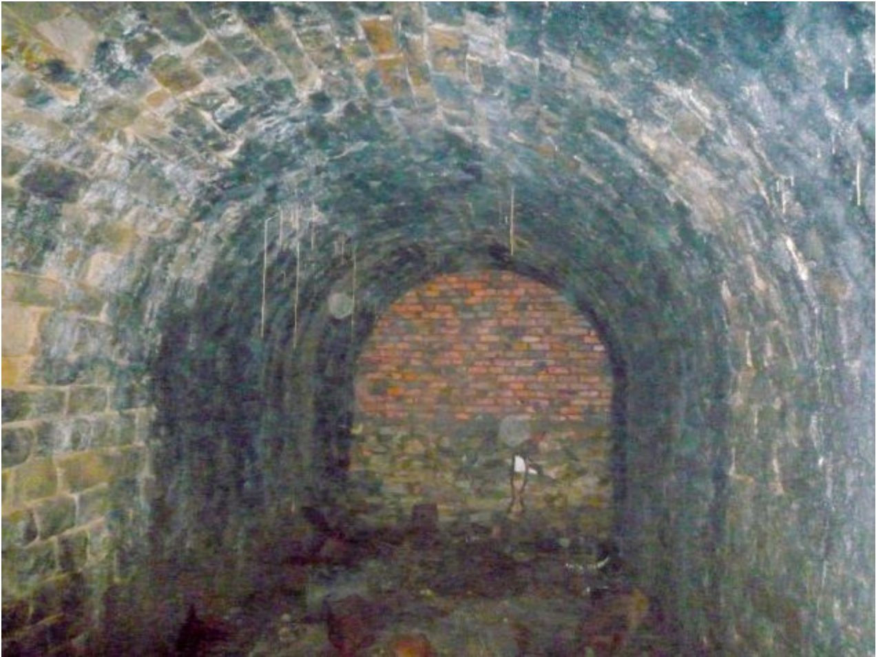
Historic: The tunnel is connected to the Butterley Gangroad, a horse-operated railway built in 1793, by the Butterley Company, a large local engineering firm
